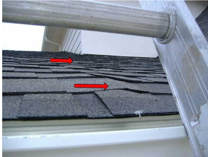
1. Excessive construction gap at the rear lower roof transition.
